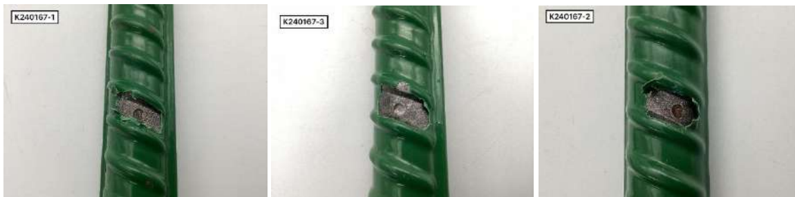
Details disbonded area
