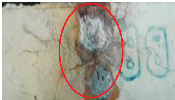
Fig 6. Outside Surface of Concrete Block with Black Bar
