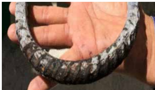
Fig 8. The U Bent Portion of Steel Bars Suffered Heavy Corrosion
